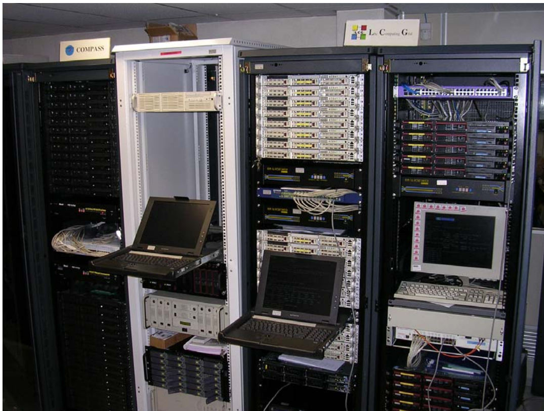
Figure 6.1: Typical GRID farm (INFN Turin Computing Centre)
