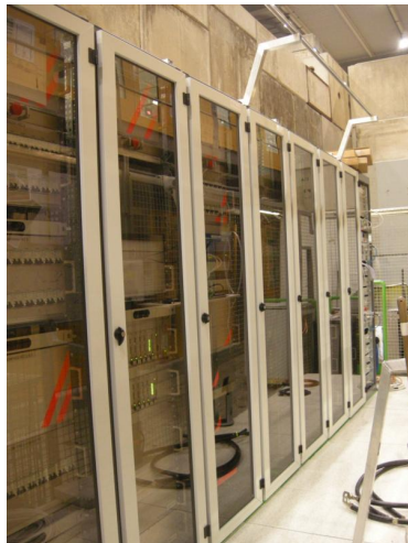
Magnet control racks.
